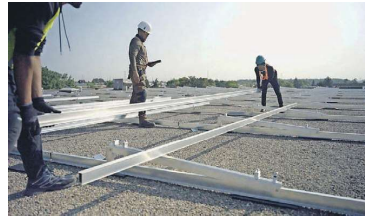
Rabba Fine Foods is currently installing solar panels on the roofs of two of the company's distribution warehouses. JOHN BREGGAR PHOTOGRAPHY
