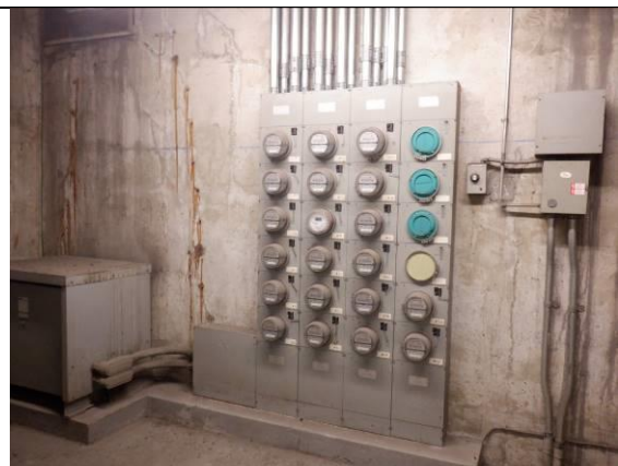
Electrical room – separate meters
